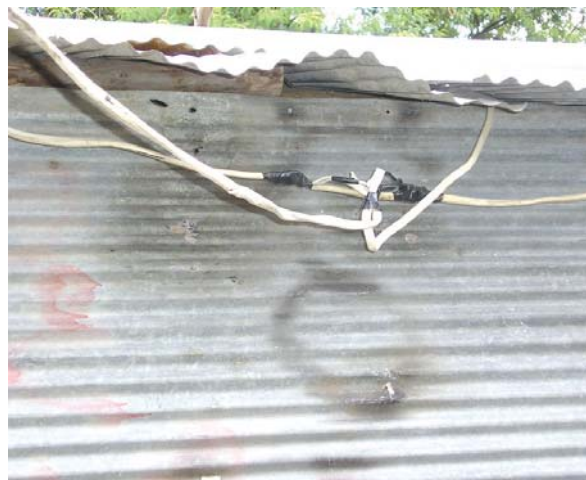
Exposed wiring on tin roof of migrants living quarters
